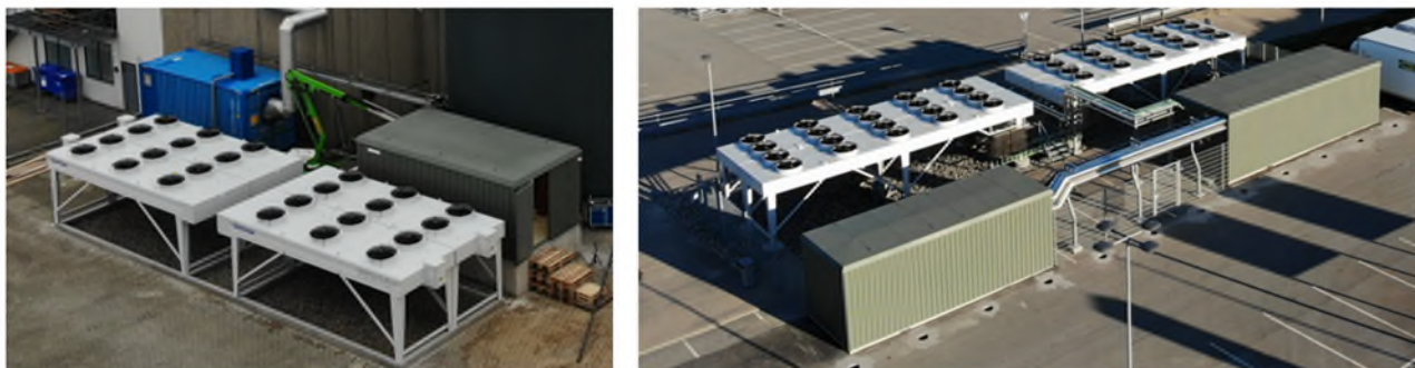
Figure 14: The Havneby installation to the left and the Alborg installation to the right.
