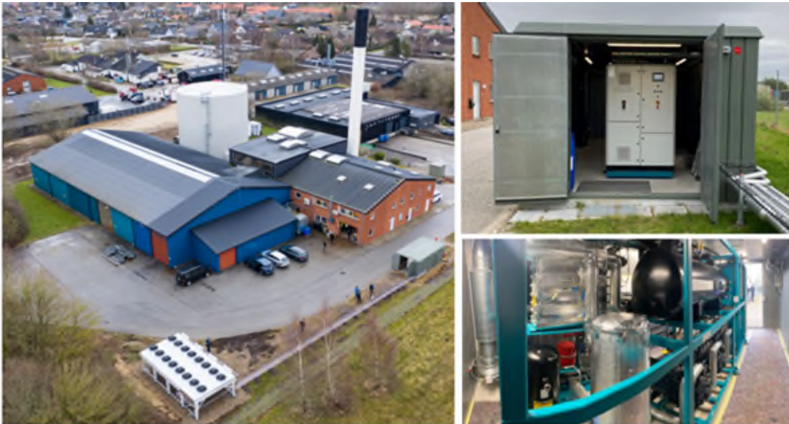
Figure 45: 600 kW field test unit in Harlev.
