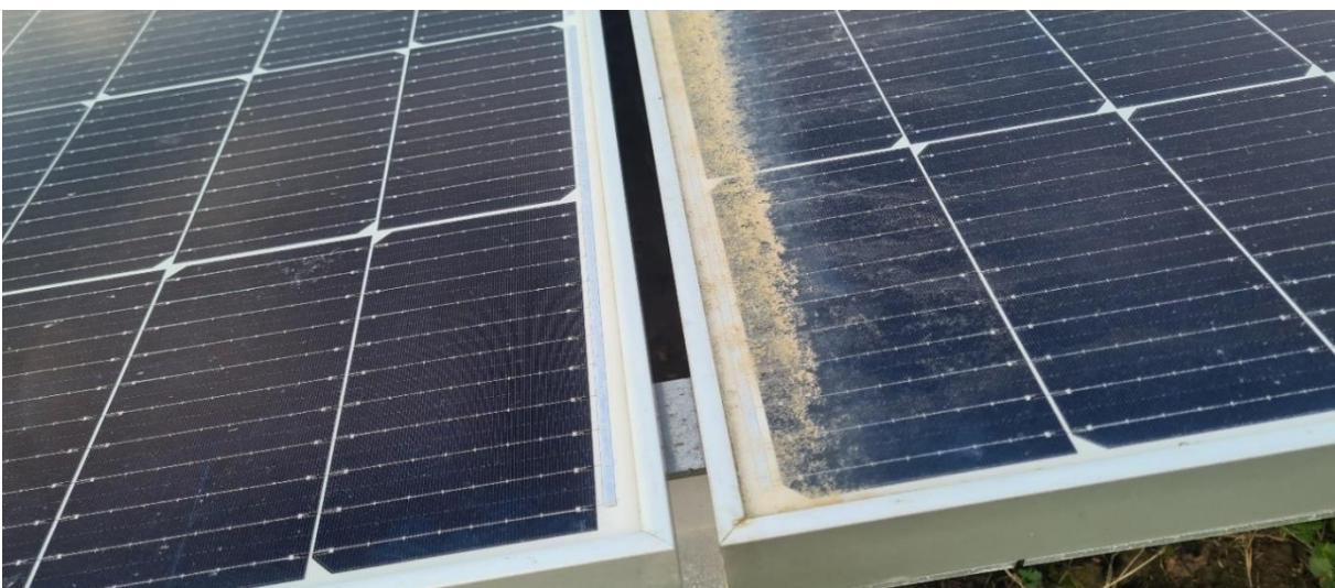
Figure 21. Example of dust accumulated near the lower edge frame of a PV panel
