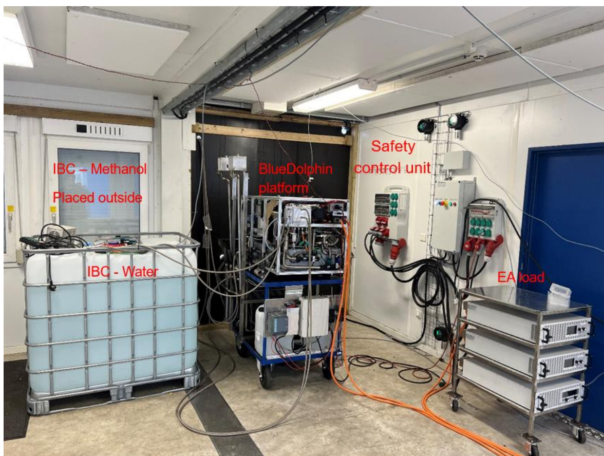
Figure 21 Inside of the test container
