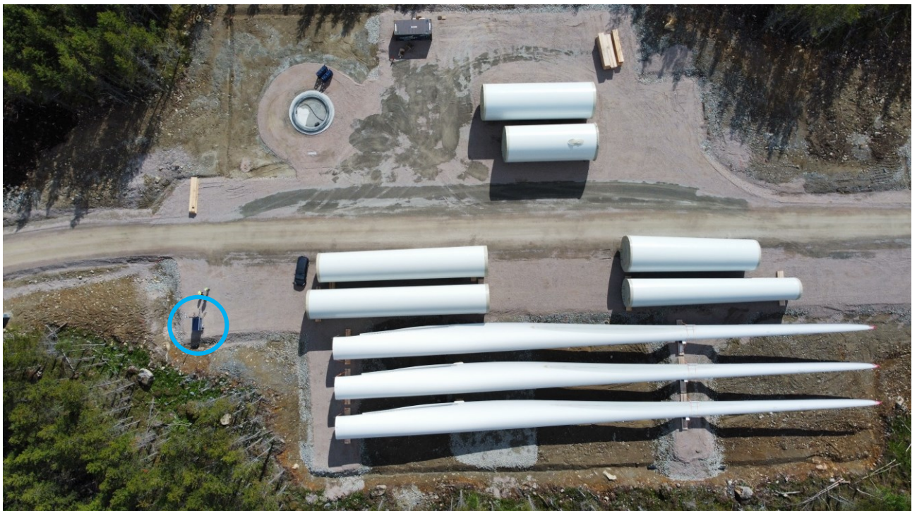
Aireal view of the position of the solar trailer on a wind turbine hardstand
