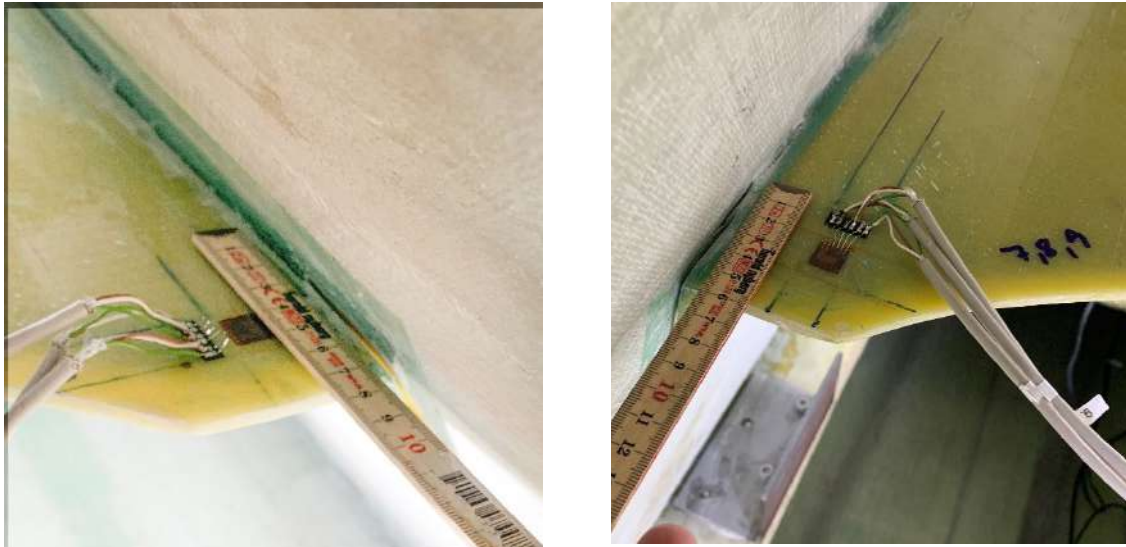
Figure 19: Damaged aft shear web bondline on the Pressure Side (left) and damaged bondline on the Suction Side (right).
