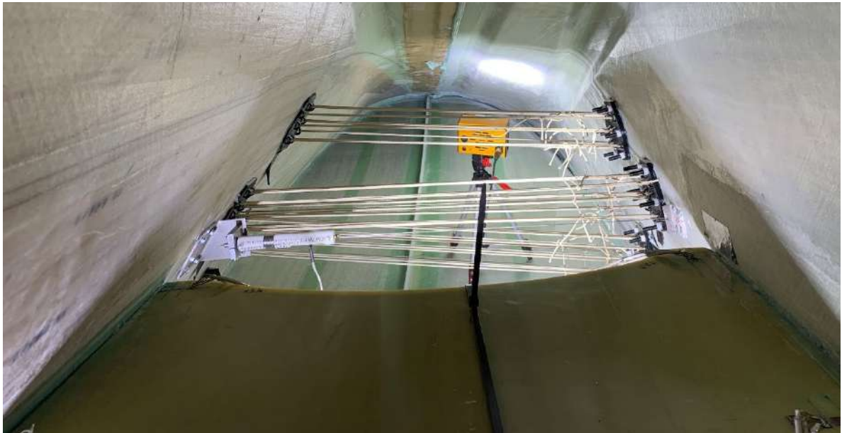
Figure 22: The RTZ Solution™ installed inside the 15m blade cutout of the SSP34m blade.
