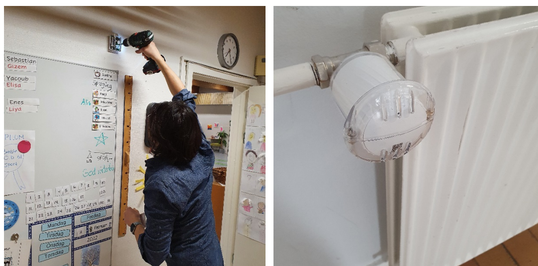
Figure 13 Left: Installation of MClimate indoor sensors and notifiers. Right: Mclimate LoRaWAN VICKI smart thermostatic valve head with anti-vandalism plastic cover mounted on thermostat
