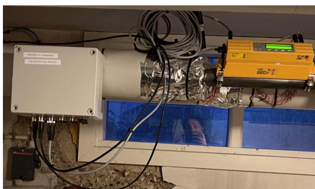
Figure 14 Picture of the first installation of UpSmartering's system at Borgerskolen in Høje Taastrup municipality. On the lefthand side you see UpSmartering's data harvesting box. The yellow device on the right side is the power meter installed to the district heating piping.
