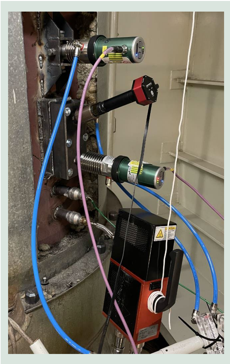
FIGURE 16. In-situ installation with extractive probe installed from the reference sensors.
