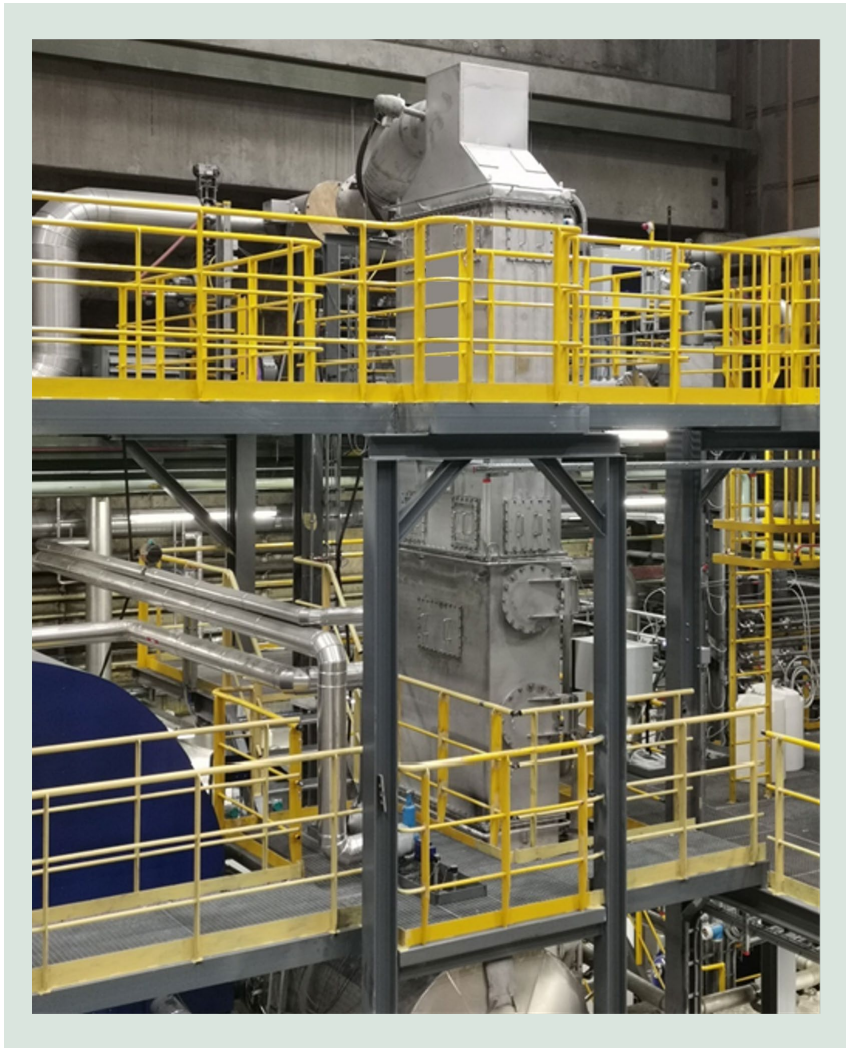
FIGURE 2. Wet ESP in the Alfa Laval Test and Training Centre.
