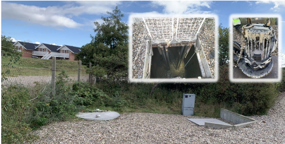
Figur 29. Pumpestation, Havneby Rømø (submerged).
