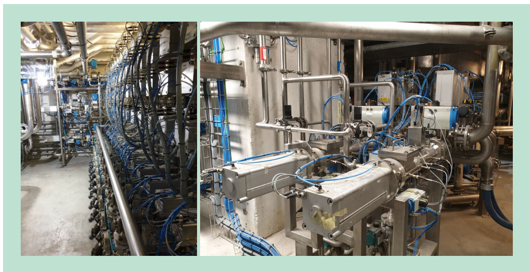
FIGURE 8. Details of renovated factory with filter station, station with pipes assigned for filling station and pipes prepared for optimal cleaning.
