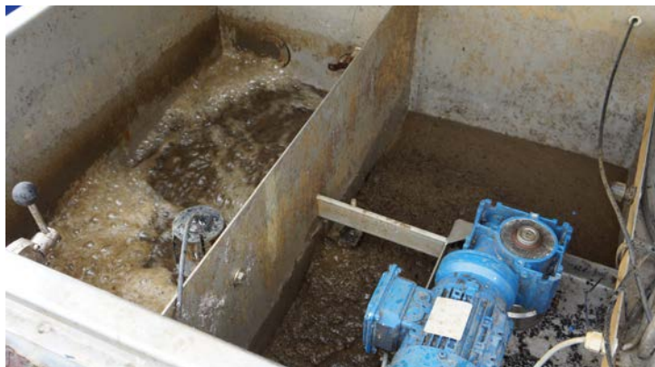
Figure 5: One of the two membrane lines in operation
