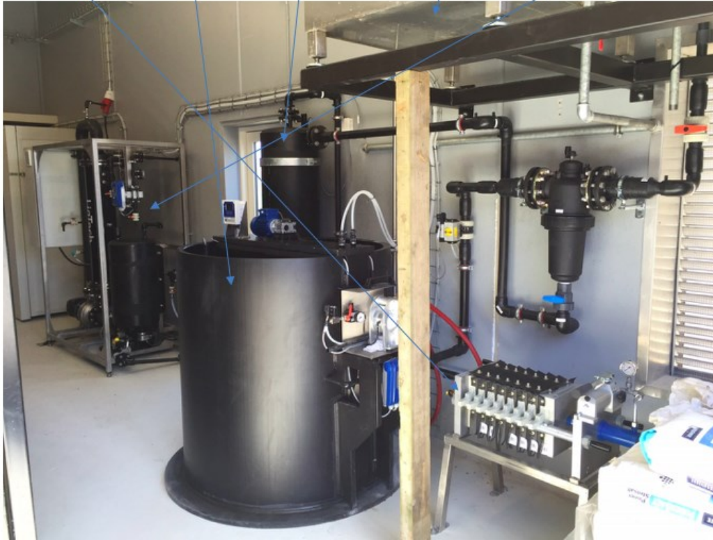
Figur 4: The functional plant in Vestervig
