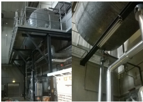
FIGUR 3-6 RO LAGERTANK, HVIDOVRE HOSPITAL
