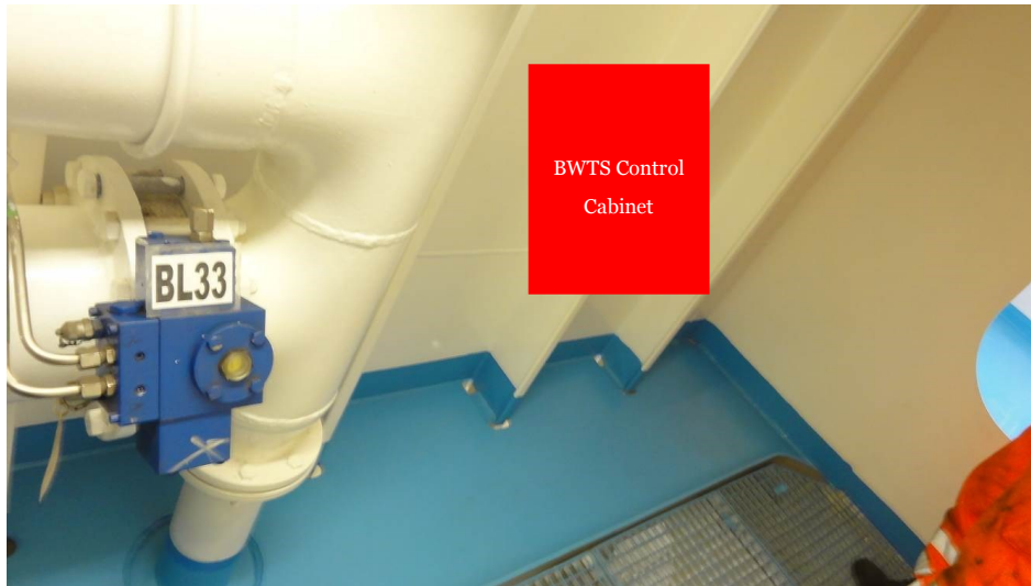
Picture 17: Location of BWTS control cabinet
