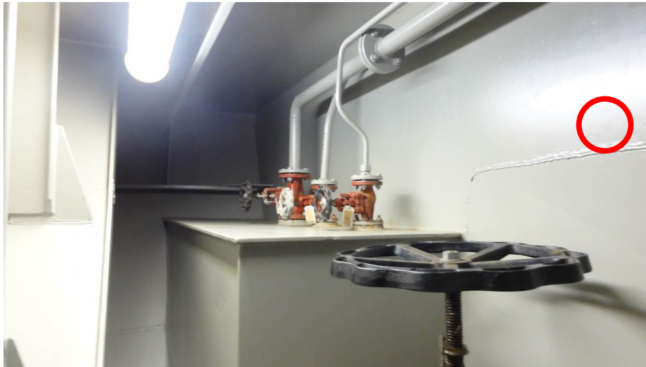
Picture 145: Piping penetrating bulkhead from engine room in Lower Starboard Pump Room
