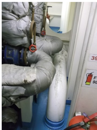
Picture 9: Limited available space in pump room (From Boringia Swan)
