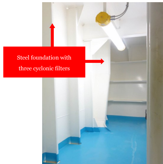
Picture 112: Position of three cyclonic filters in Upper Starboard Pump Room
