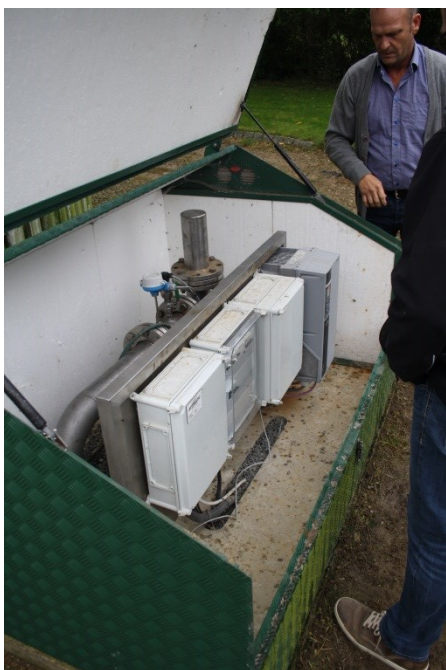
Figur B5-1 Pumpestation.
